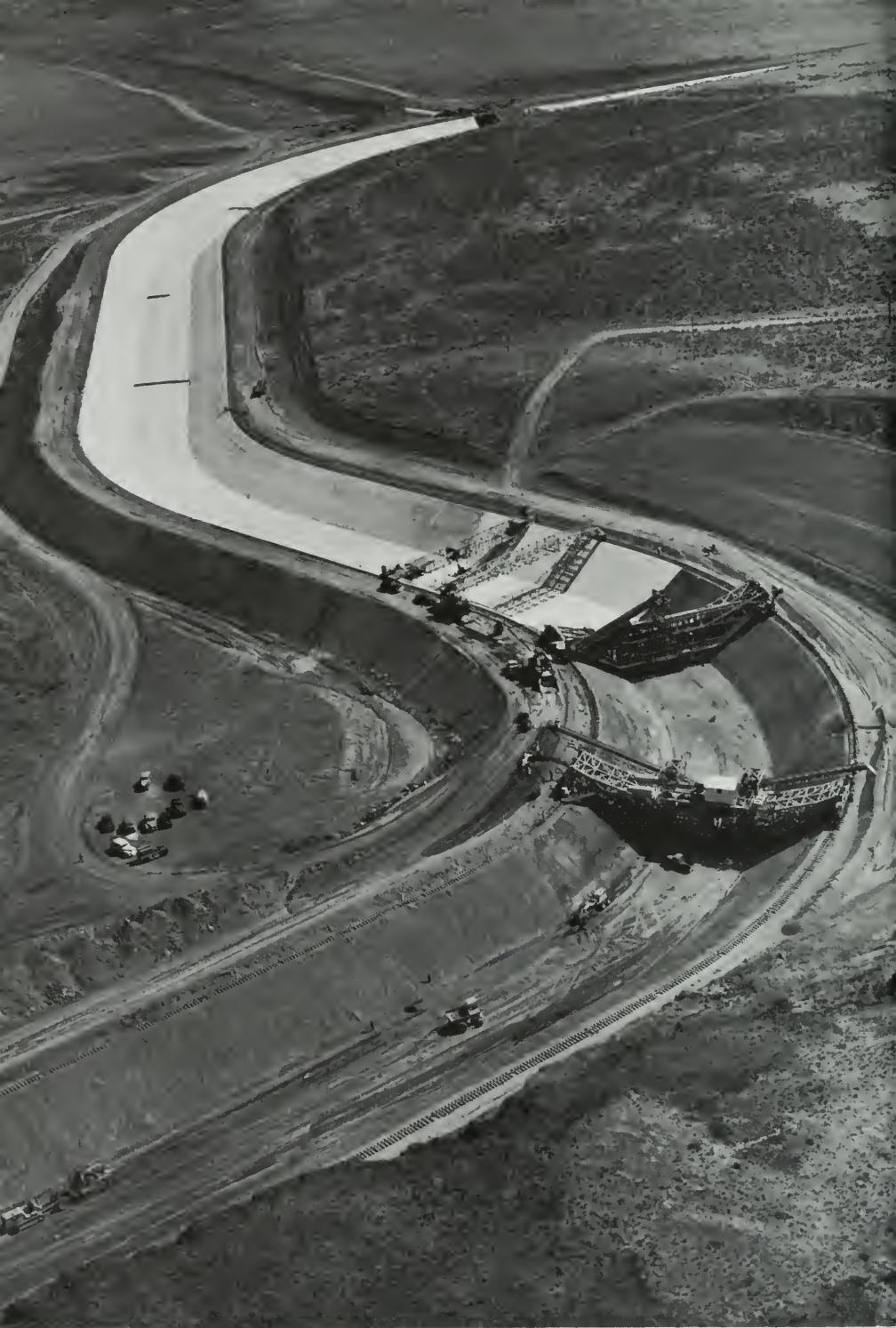
Lining with concrete the main canal of the Columbia Basin Project in Washington.
